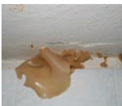
fungi on walls
