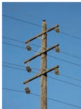
Figure 19.15 (b) – Wooden electrical posts
