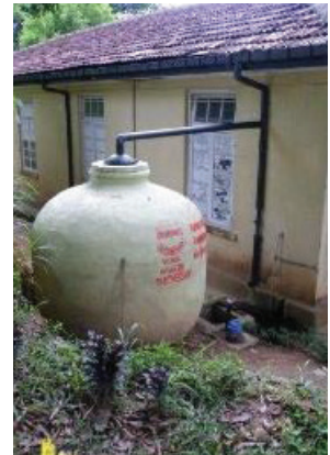
Figure 13.10 – A device set up in a house to collect rain water
